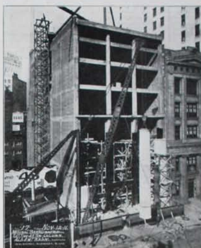
Work in progress on the National Bank of Commerce, Fort Street West, Albert Kahn, architect.
