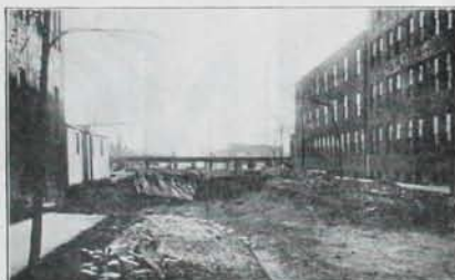
Grade separation work, Twelfth Street and Michigan Central and Grand Trunk tracks, Detroit.
