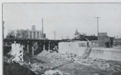
Grade separation in progress at Wabash Avenue and the Michigan Central and Grand Trunk tracks, Detroit.
